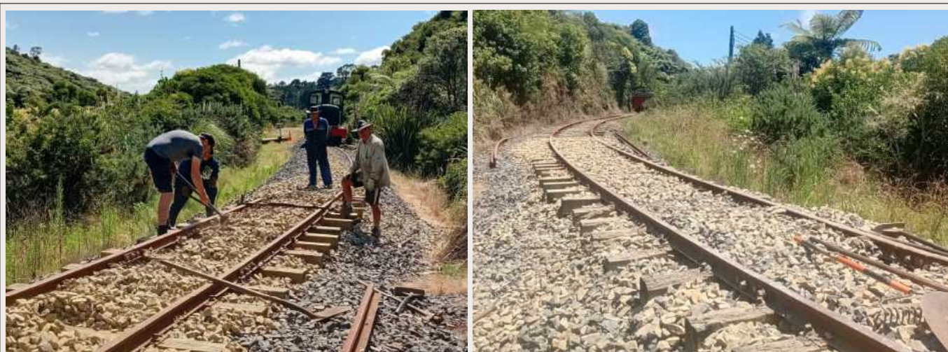
Above: Sandfill track work in January – lifting of the curve completed (Mike A)
