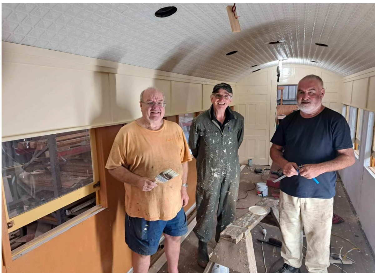
Over 3 weeks Richard E, Rob B and Dave M & Russell W (not in the picture) painted the walls and ceiling in the recent work on A1477,
