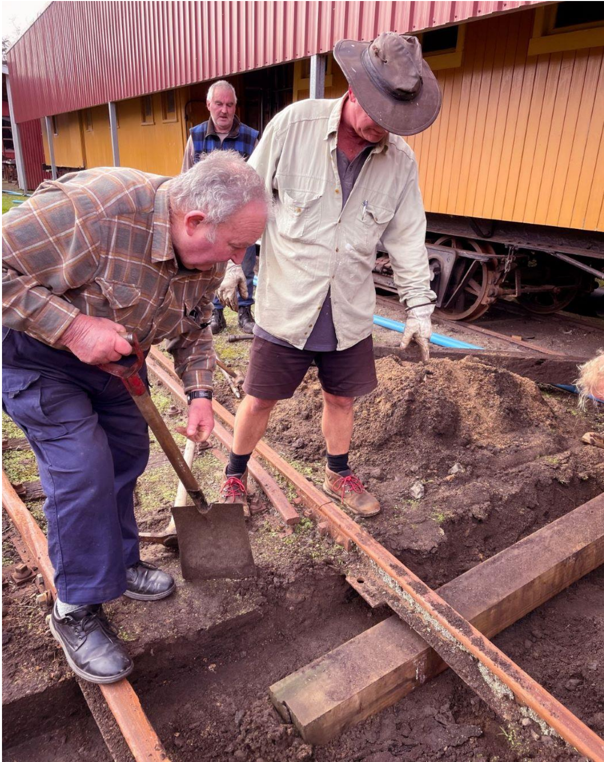
CJ. JS & DM at work replacing a sleeper in the yard (G. Coker)
