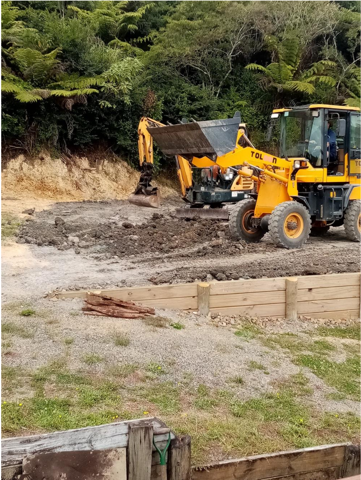
The digger placing spoil where the hall used to be (Russell Webb)
