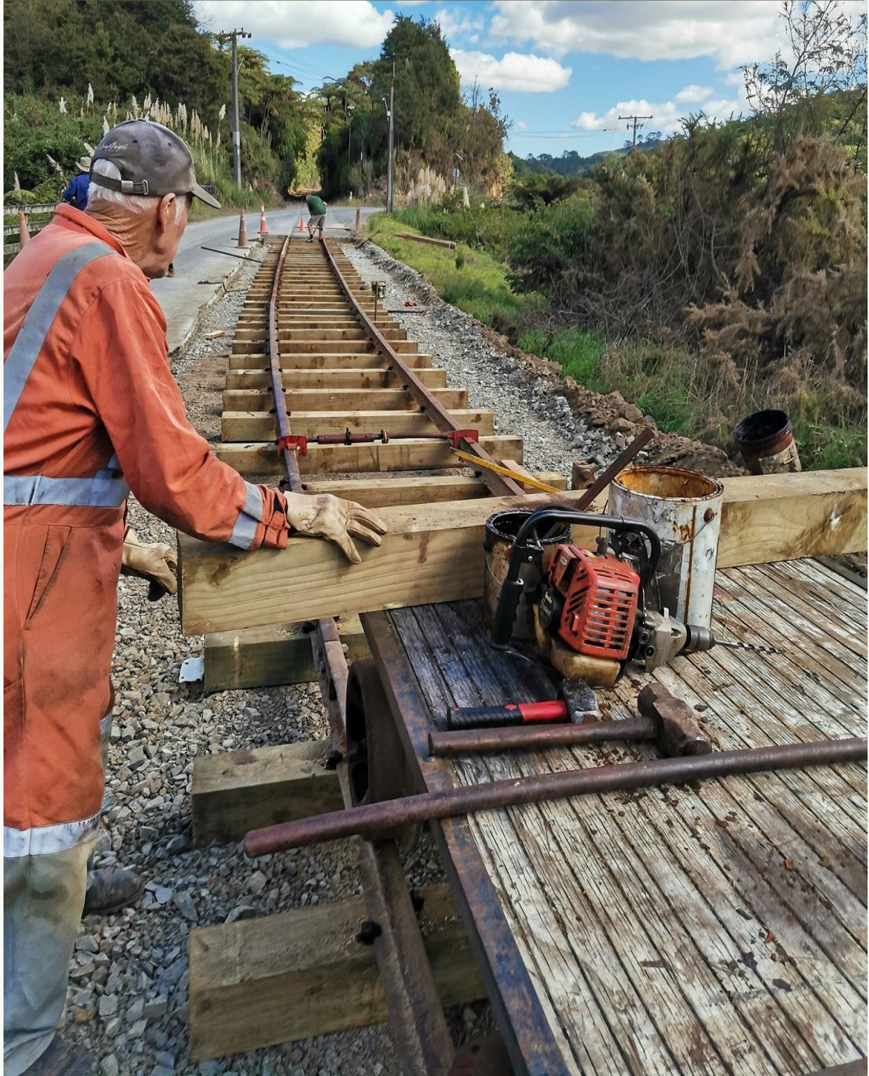
Maarten surveys the newly laid line at the top of the yard— April 2022 (T. Willmot)
