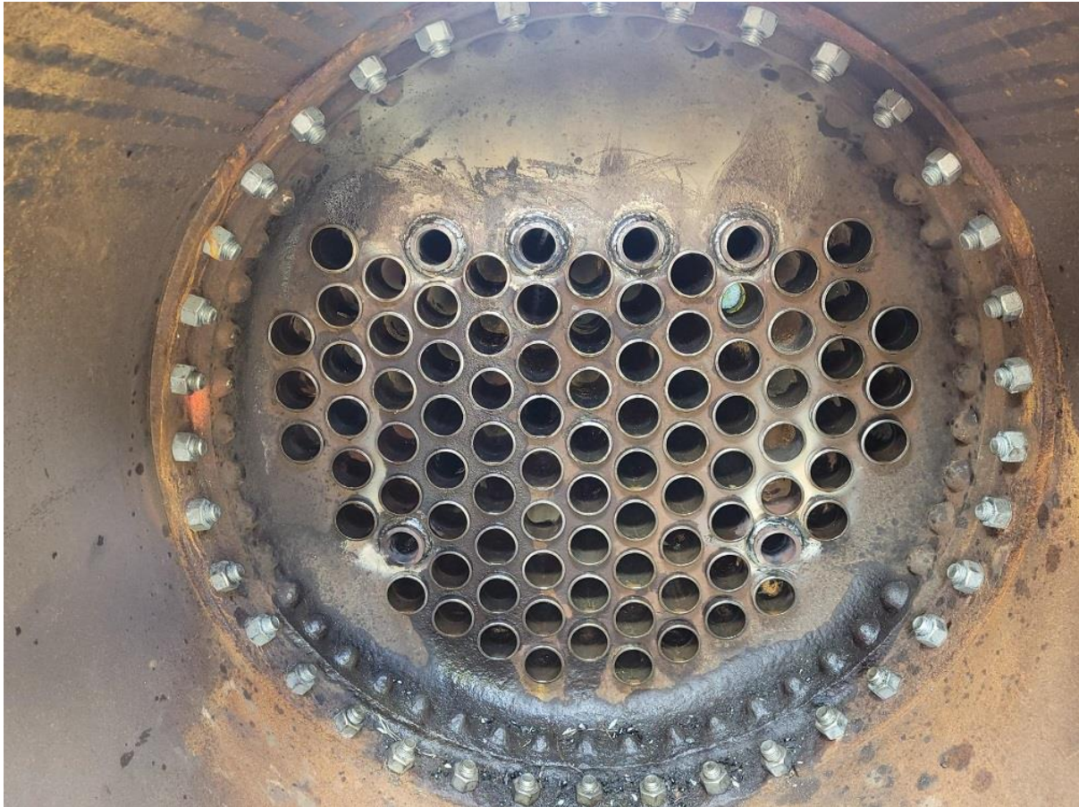
Heisler tubes in position at the smokebox end (Alastair McIvor)
