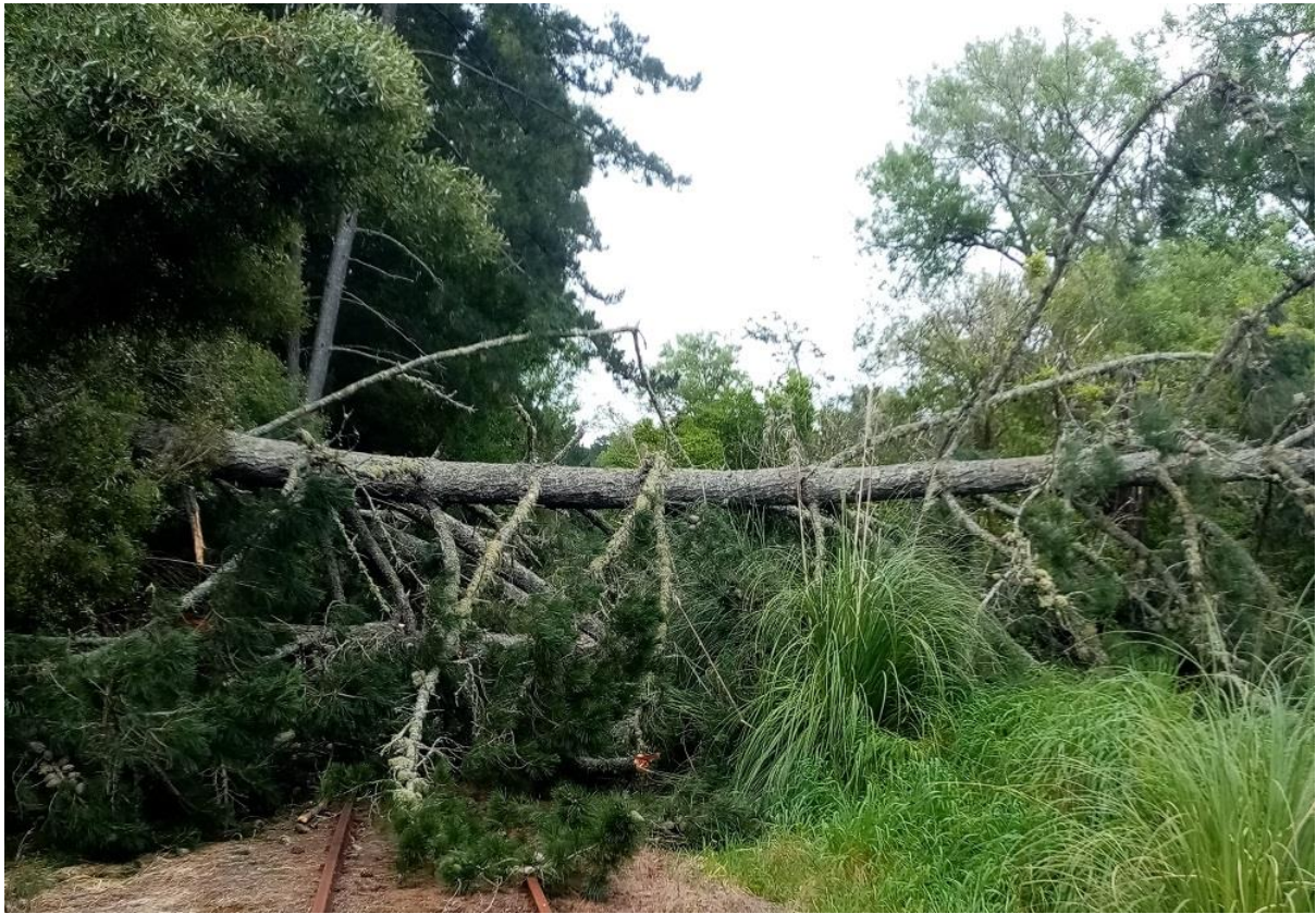
Tree over the line near Glen Afton in early November (R. Webb)
