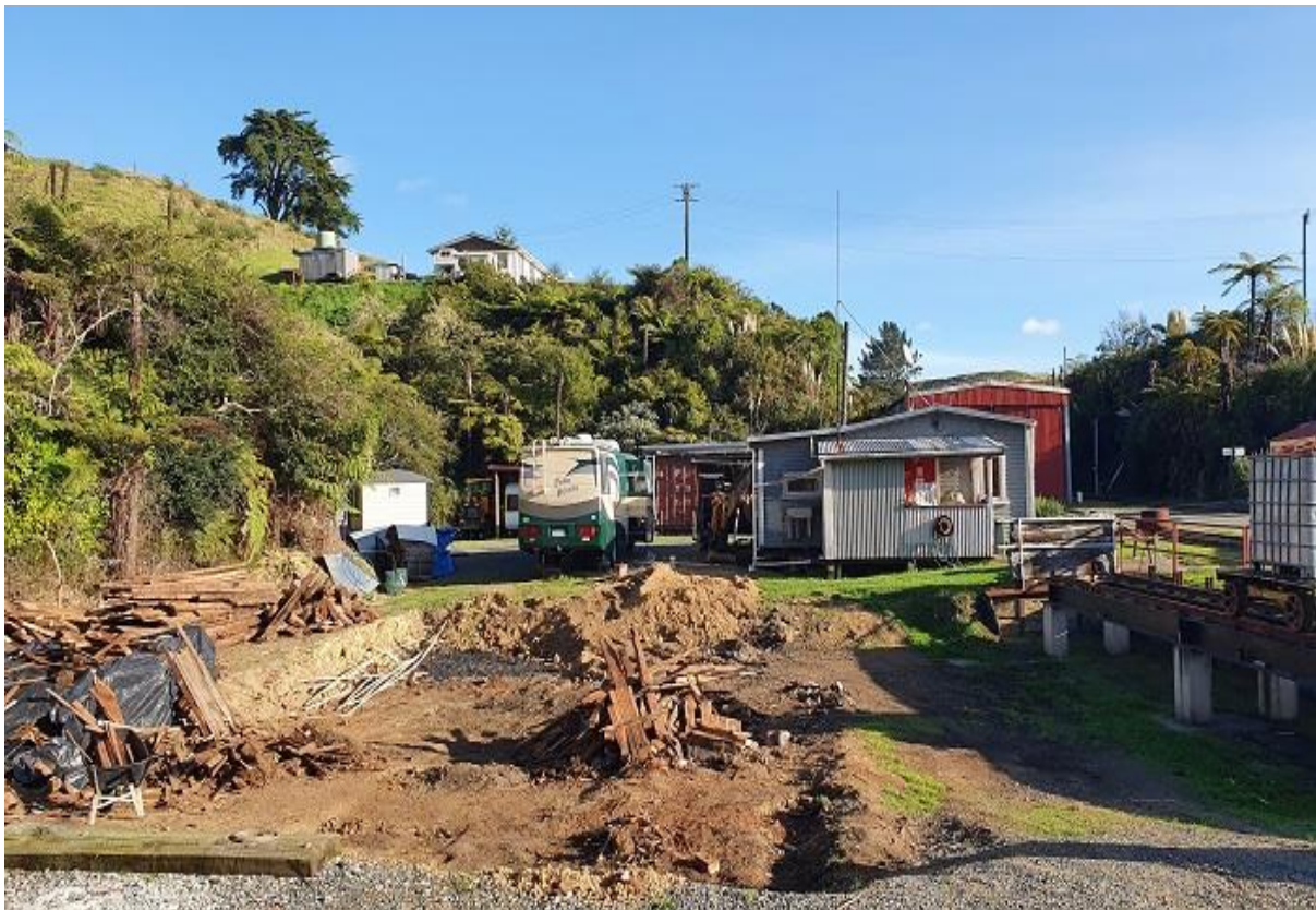
The PJ Hall area after the Hall floor had been removed (R. Ellis)
