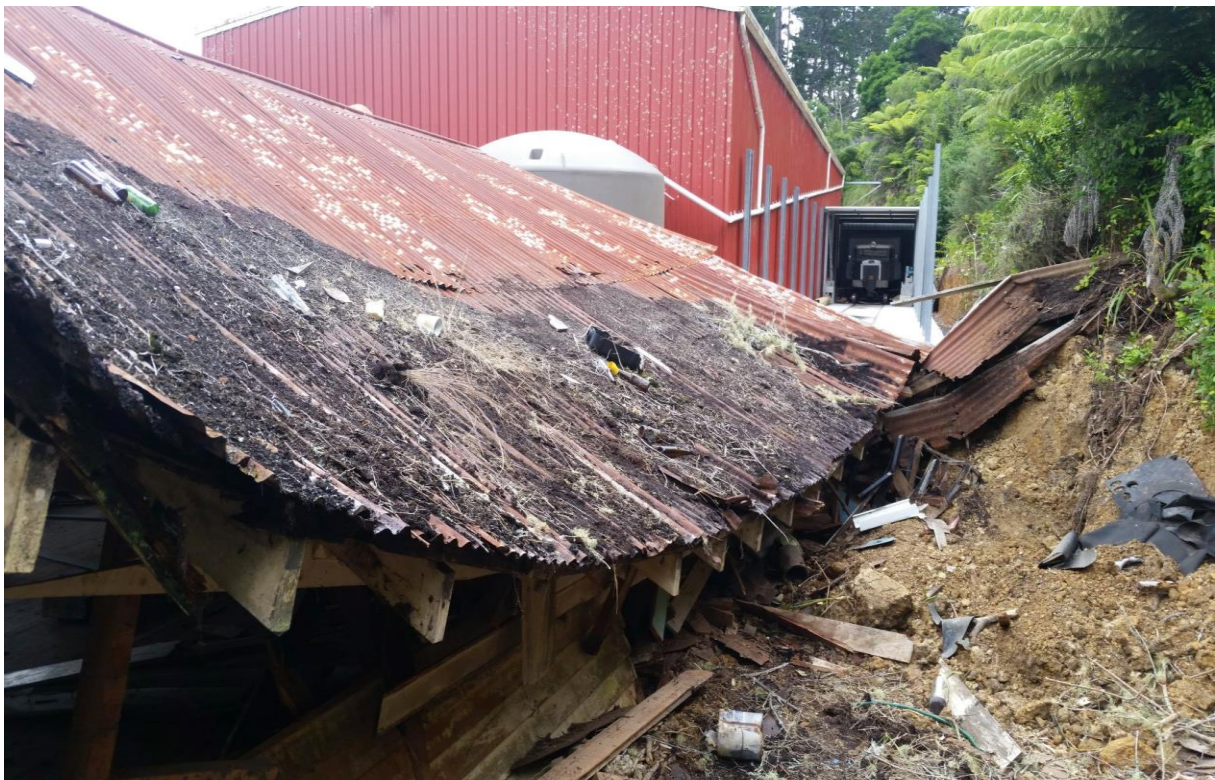
Remains of the hall roof with the new lean-to for the woodwork shop in the background plus a distant jigger (Rob Beaumont).
