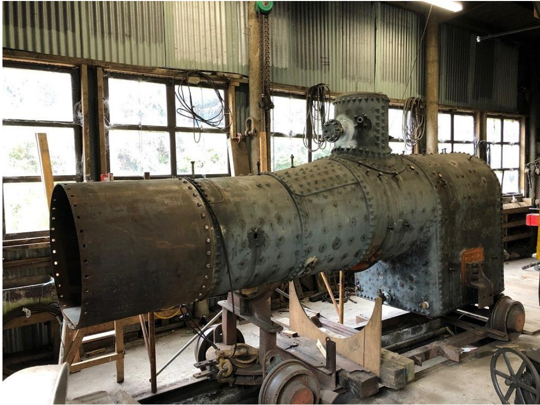
The Climax boiler is just about completed. Note the new steam take-off on the dome (image: Chris Mann)
