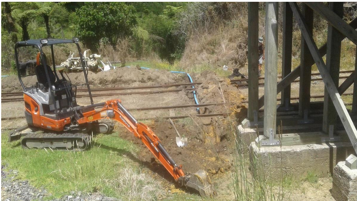
Bruce McLuckie recently got a machine to dig the trench for the water supply to the new loco water tank (Photo: B. McLuckie)
