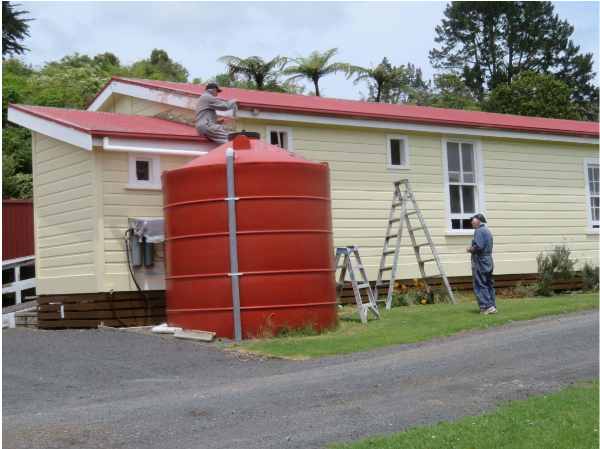
Rob & Sue Beaumont replace the stolen CCTV cameras on the newly painted station. Dave Mann also did considerable work on this. (R.Ellis)
