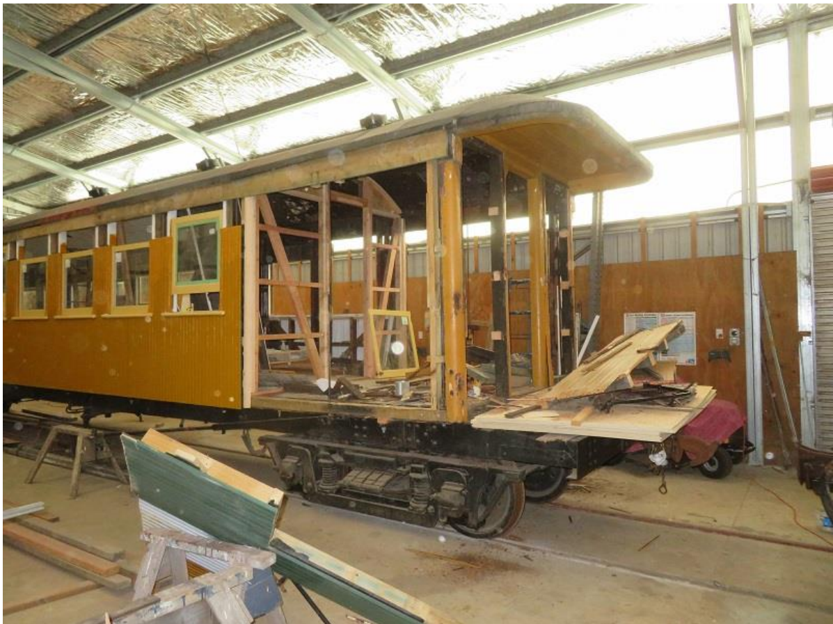
A1477 progress – a new bulkhead frame can be seen – thus allowing a much larger balcony so passengers can enjoy the view in the open air – Chris Mann is working on the engineering modifications (R. Ellis)
