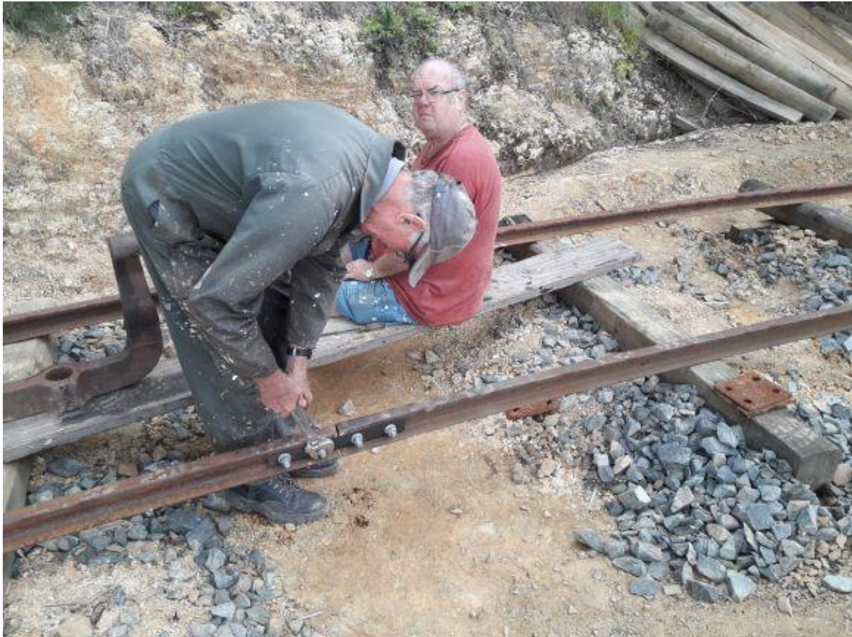
Rob Beaumont wields a spanner on the new siding for the battery electric loco whilst Richard Ellis “supervises” (T. Townsend)
