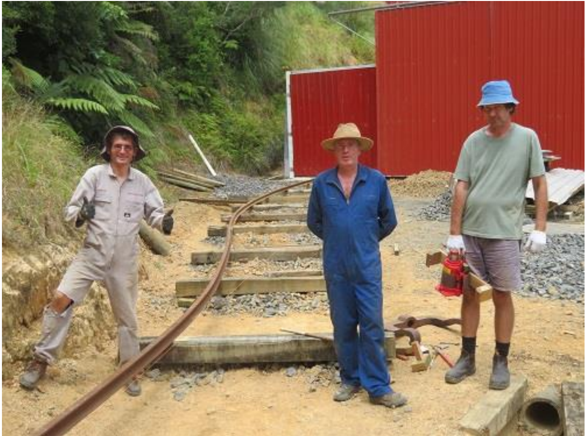
Robert, Alun & Trevor lay the sharply curved battery electric loco siding in February 2019.....(R. Ellis)
