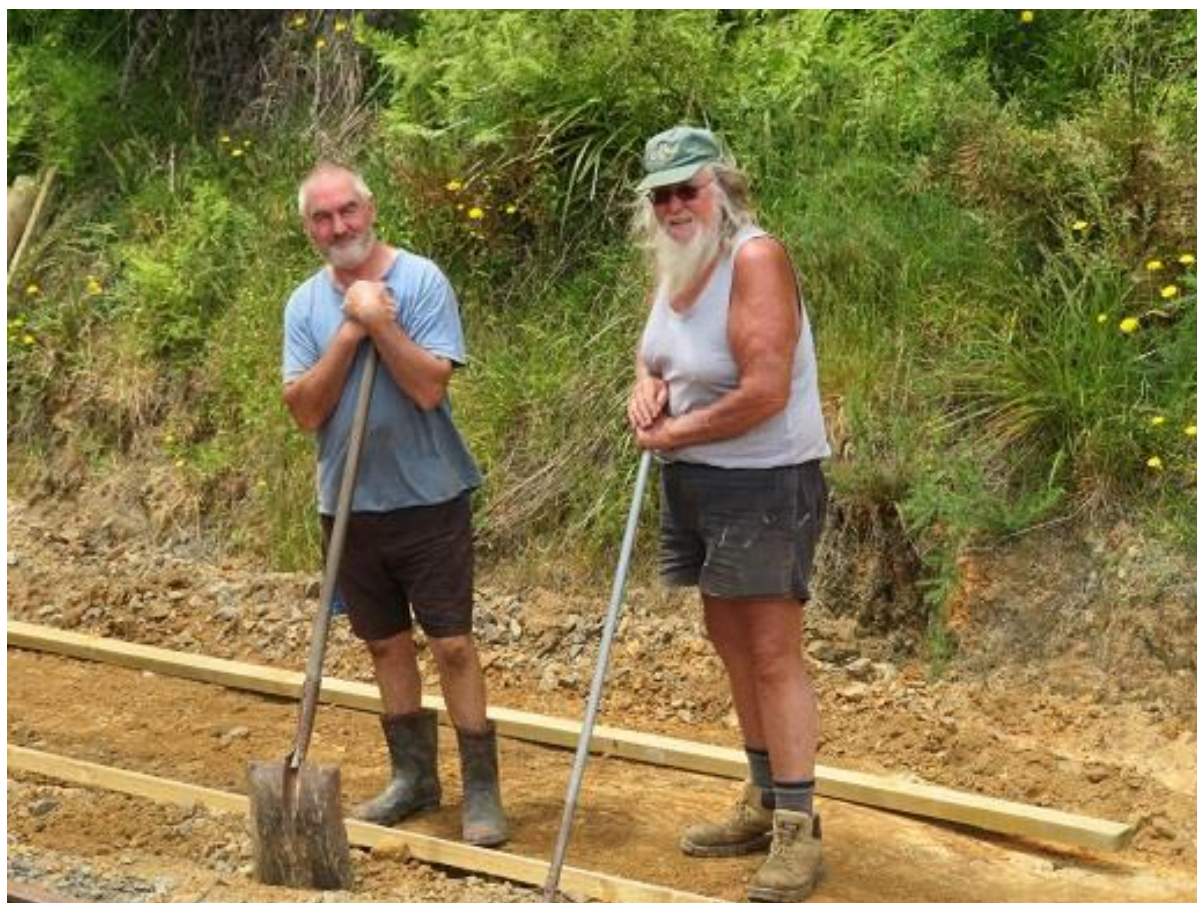
Dave & Russell clear the way for the new siding to the battery electric loco shed – bring your shovel in 2019!.....(R. Ellis)
