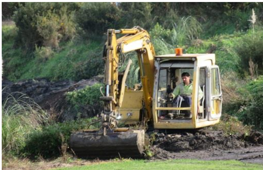
Dean McQuoid working on reinstating the track all the way to Glen Afton – here seen at the future Glen Afton station site (Richard Ellis)
