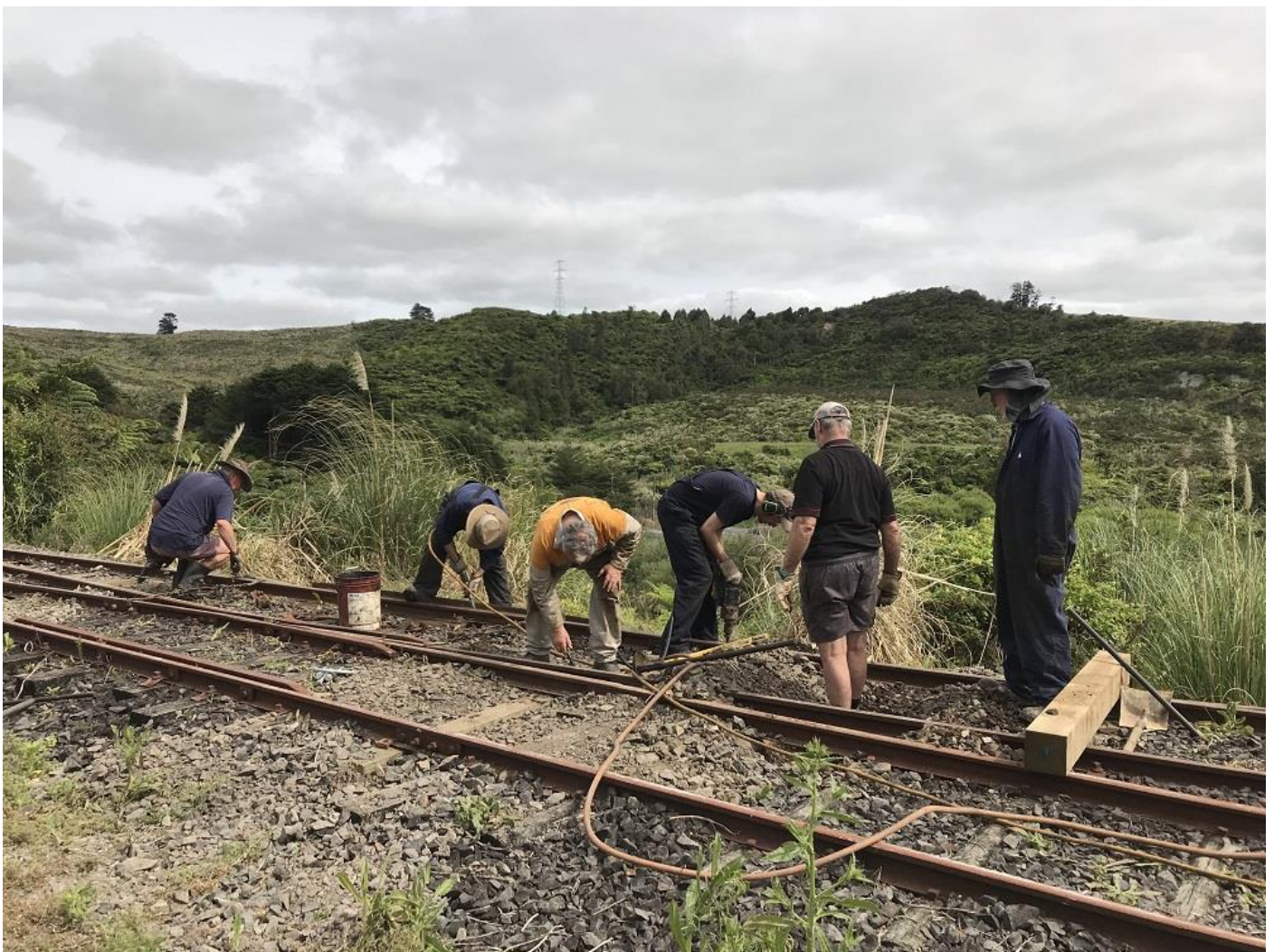
Members working on the track – an essential task to keep the railway functioning...
