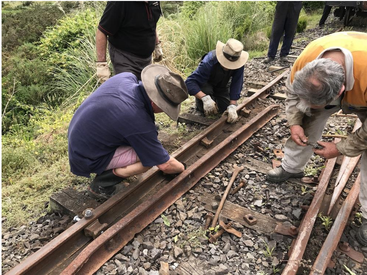
Members sort out check rail issues at Rotowaro during the recent working bee...
