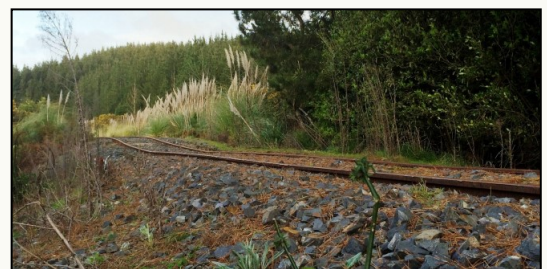
The slump below Hangapipi Road (Image: E.B.)
