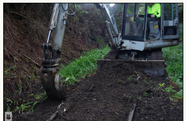
DCM machines at work! Top: at the slip with David and the tipping wagon. Above: Watercress Cutting. (Images: G.C.)
