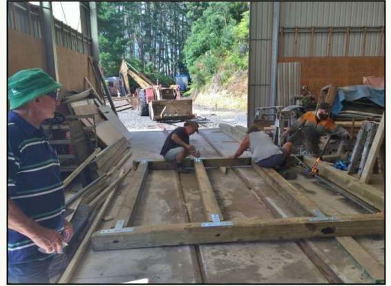
The last of four water tank stand pieces being assembled (Image: E.B.)
