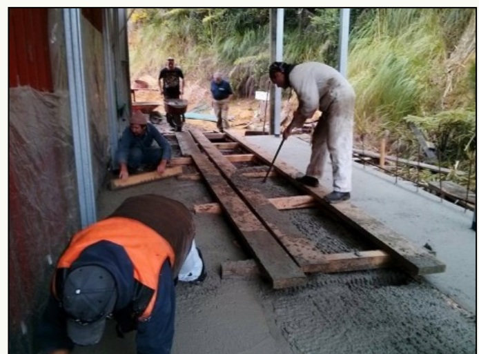
The big (little) pour as Lindsey put it, made far easier by some help from the CW crew CJ brought along. Photo: Lindsey McLeod
