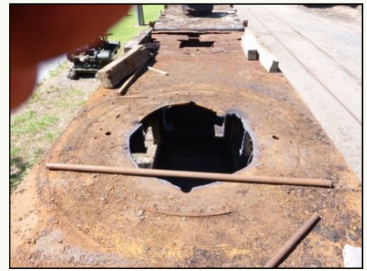
The former location of Crane 256's main pivot
