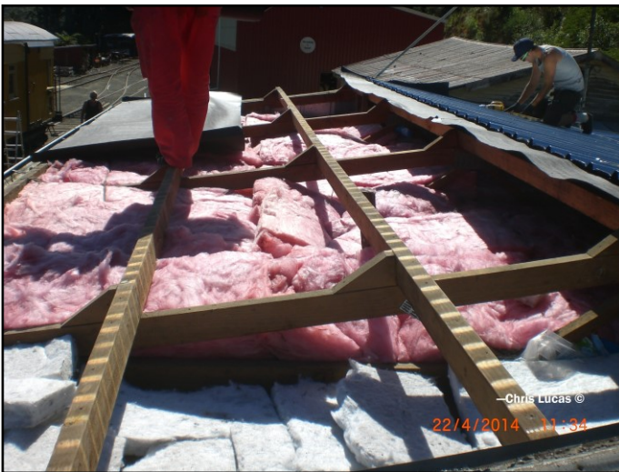
Here we have the new roof being put on the shanty. The new insulation should be of great benefit to those who stay in it on cold winter nights.
