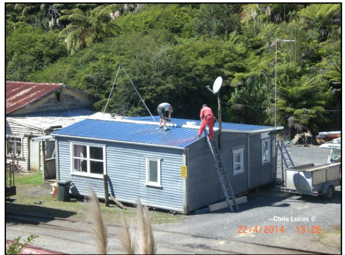
Here we have the new roof being put on the shanty. The new insulation should be of great benefit to those who stay in it on cold winter nights.
