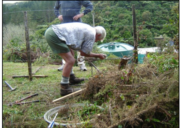
Here we have Kelly Gifford and Ian Hampton (well most of them) repairing the track boundary fence. A unpleasant but necessary job. Keep up the good work.
